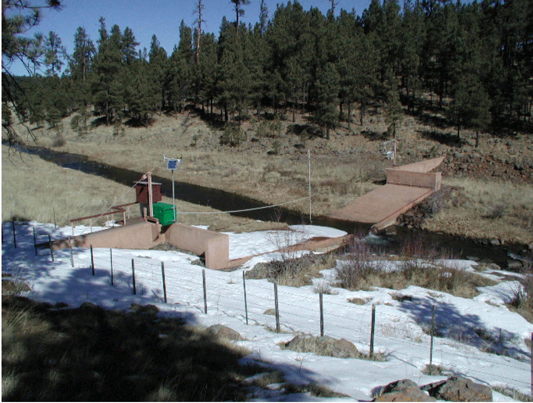
Figure 2. West Fork Black River - USFS Stream Gage with ADEQ Threshold Turbidity Sampling Station (Automatic monitoring and sampling equipment)
