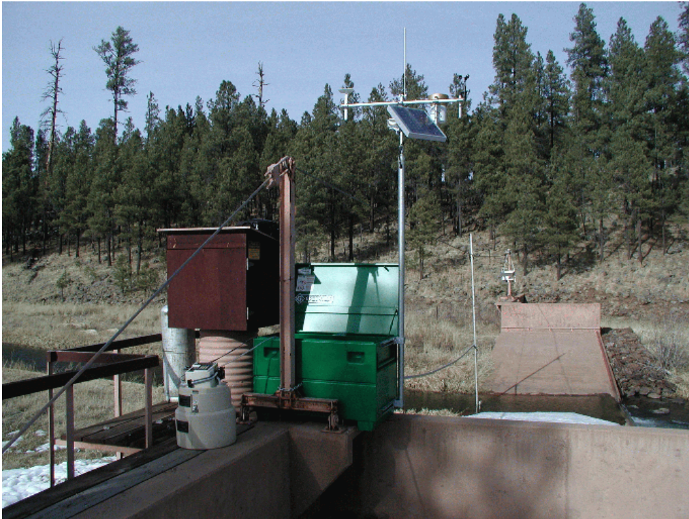
Figure 4. West Fork Black River – ADEQ Threshold Turbidity Sampling Station. The Automatic Sampler, Solar Panel, Weather Instruments and Data Logger are in/on Green Equipment Box. The Turbidity Probe and Sample Intake Boom is Suspended from Cableway at Mid-stream of Gage Weir. The WFB Station Records; Stream Stage, Turbidity, Water Temp., Air Temp., Relative Humidity, Precipitation, Wind Speed, Solar Radiation, and Soil Temp.
