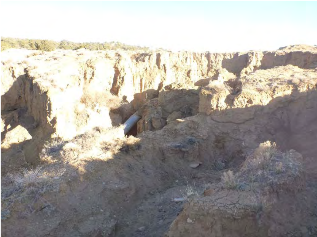
Figure 2. Downstream view of a failing water and sediment control basin. Note the outlet pipe is exposed and damaged.
