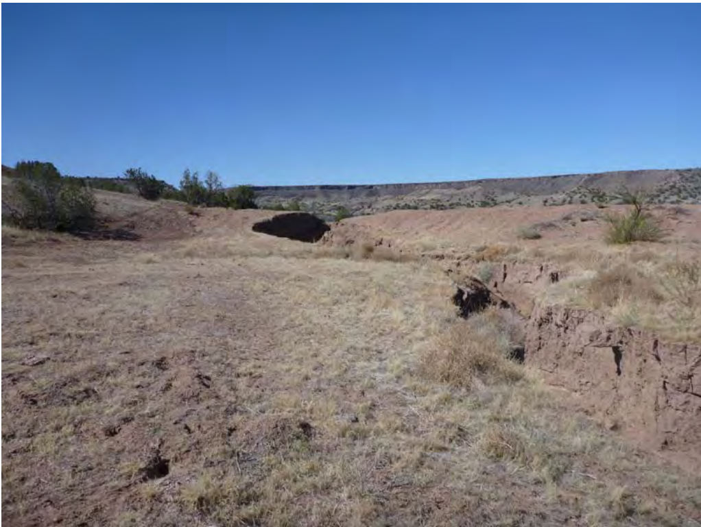
Figure 2. Photograph of the dike breach.
