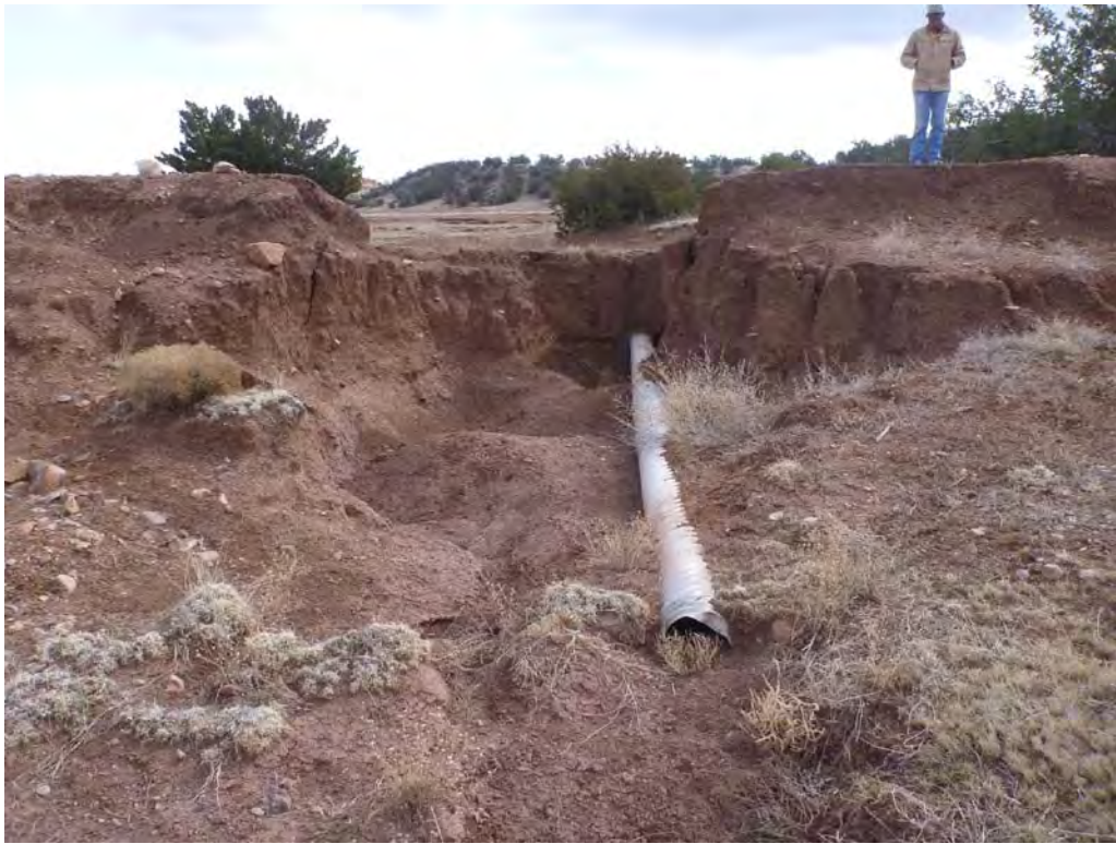
Figure 1. Failing basin with the outlet pipe exposed.
