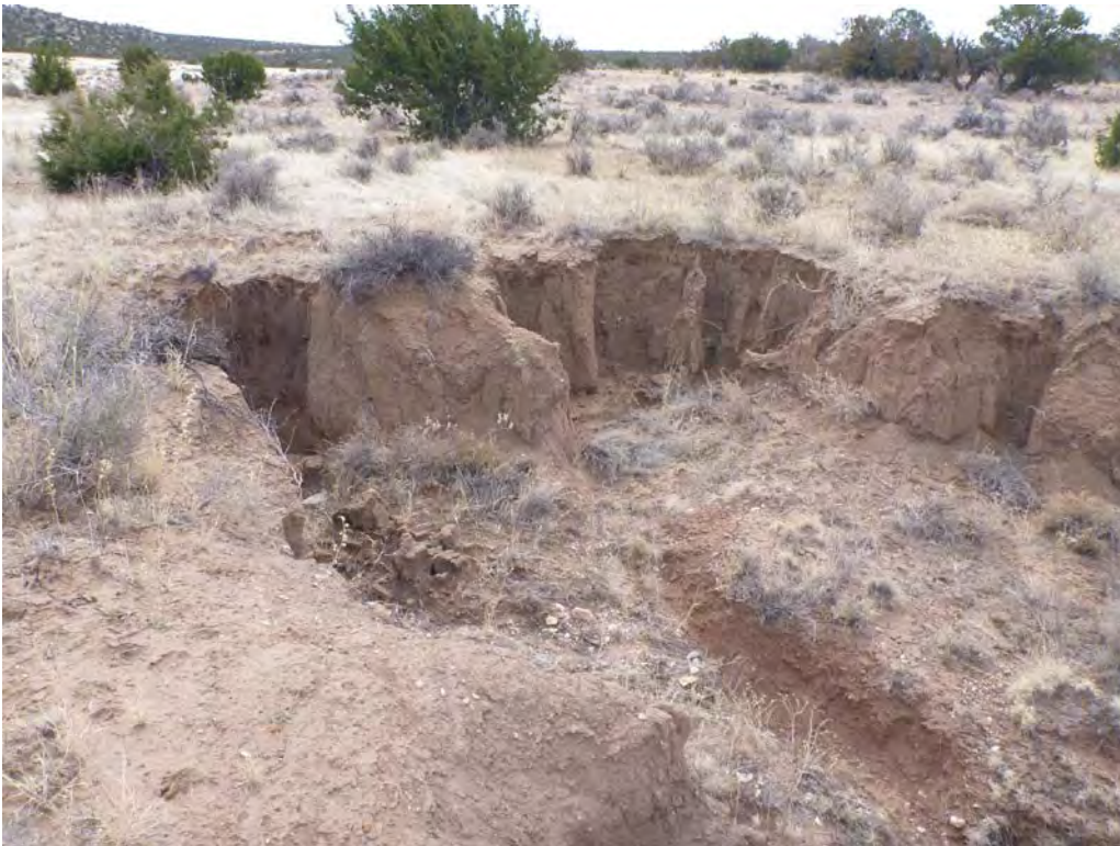
Figure 2. Headcutting to be addressed with rock lined chute.
