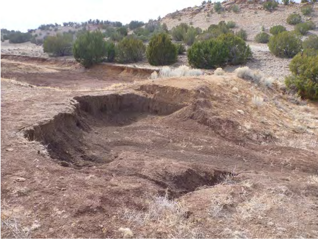
Figure 3. A rock lined chute would address the headcutting shown here, where the water has eroded through the spillway.
