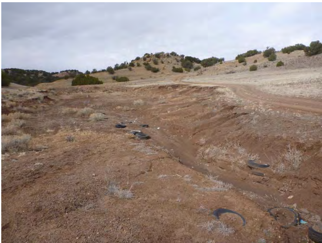
Figure 2. The basin has reached the end of its service life and is full of sediment.
