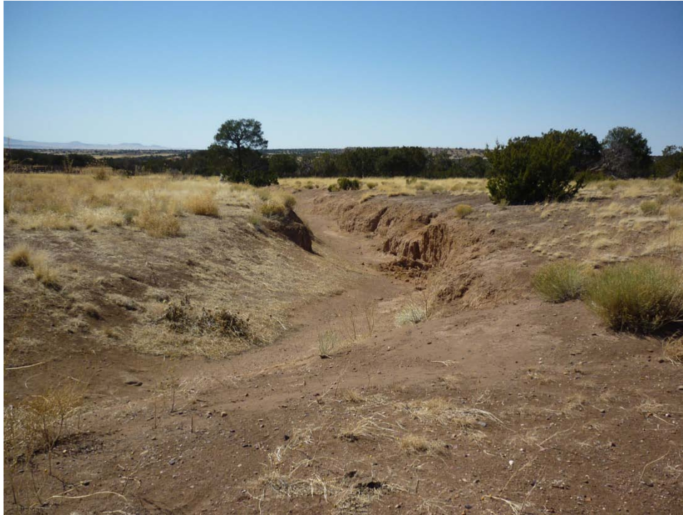
An active gully where Mr. Johnson would like to install a dike and V-mesh spreaders.
