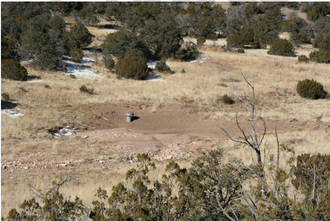
Shows a failed WASCOB that has reached the end of its service life and is potentially built in a location that has too large of a contributing watershed.
