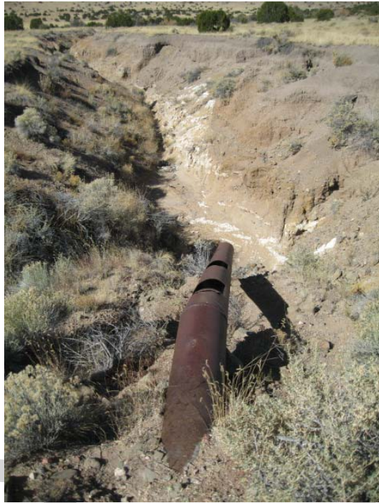
Downstream view of a detention basin; the outlet pipe is undersized and causing severe erosion.
