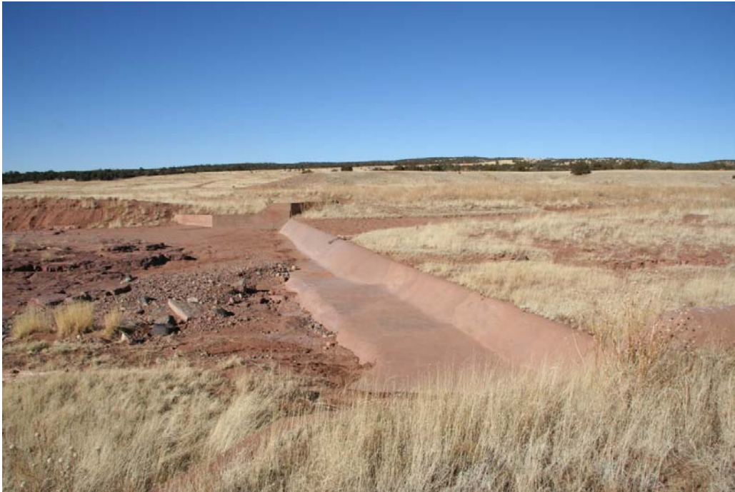
Grade-control sill has effectively controlled the course of Coyote Creek and maintained the local grade.
