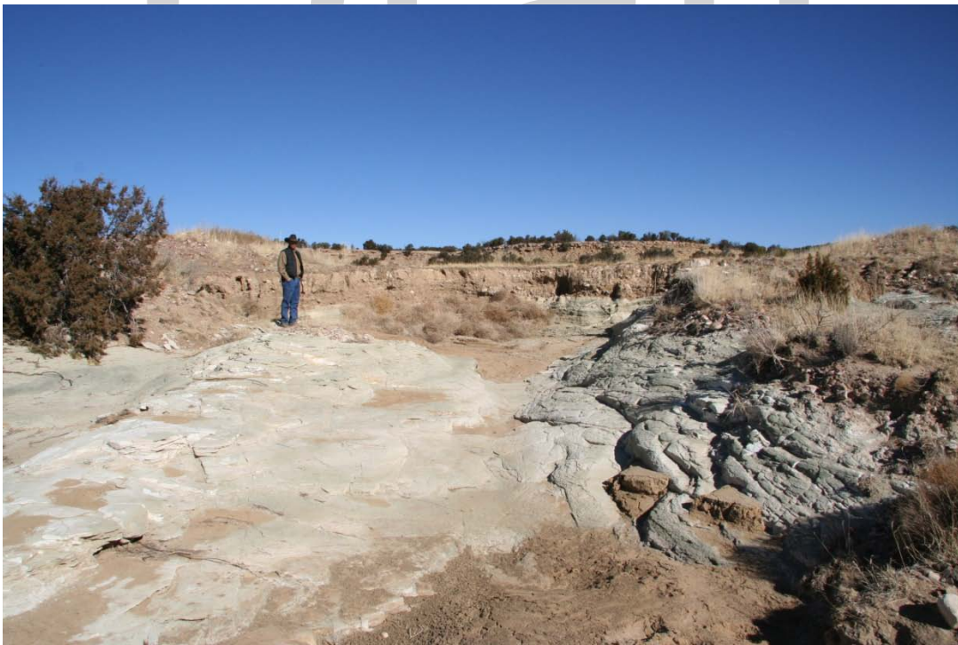
Shows an area of an actively eroding headcut.
