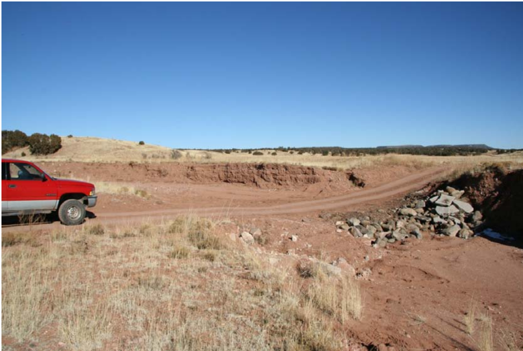
A failing grade-control structure at a road crossing on a tributary to Coyote Creek.
