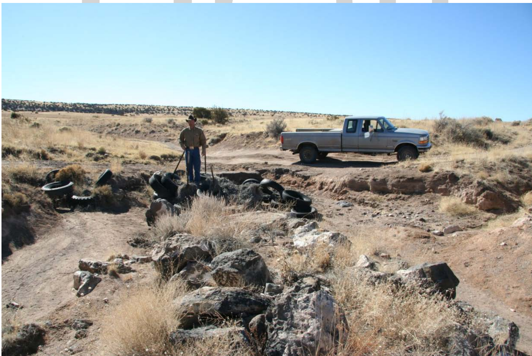
View of a failed grade-control structure made of T-posts and tires.
