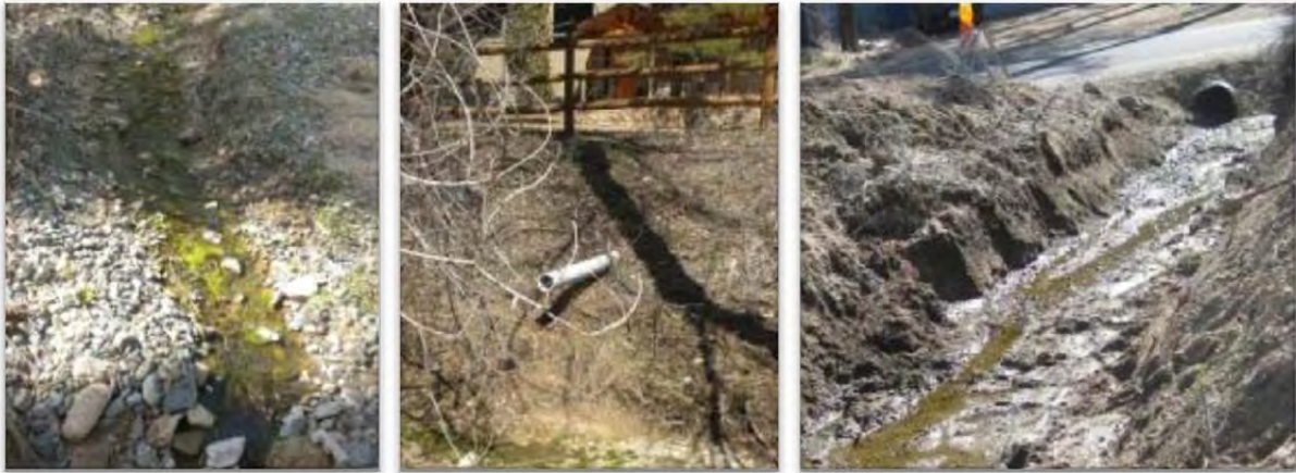
Figure 13: Stormwater Drainage Features
