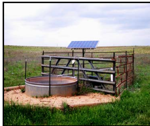
Figure 3-5: Alternative cattle watering facilities ( http://www.2gosolar.com/typical_installations.htm )
