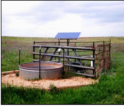
Alternative cattle watering facilities ( http://www.2gosolar.com/typical_installations.htm )
