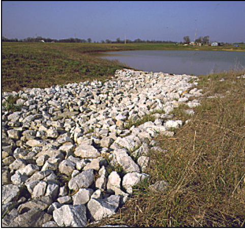
Rock Rip-Rap Sediment Control (Dept. of the Interior, Office of Surface Mining, http://www.osmre.gov/ocphoto.htm )
