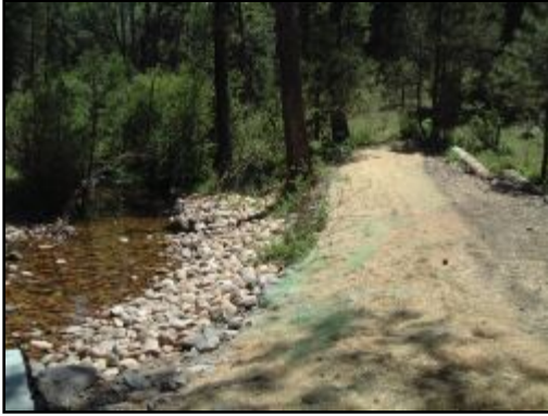
Rock Riprap and Jute Matting Erosion Control along a stream. (Photo: Lainie Levick)
