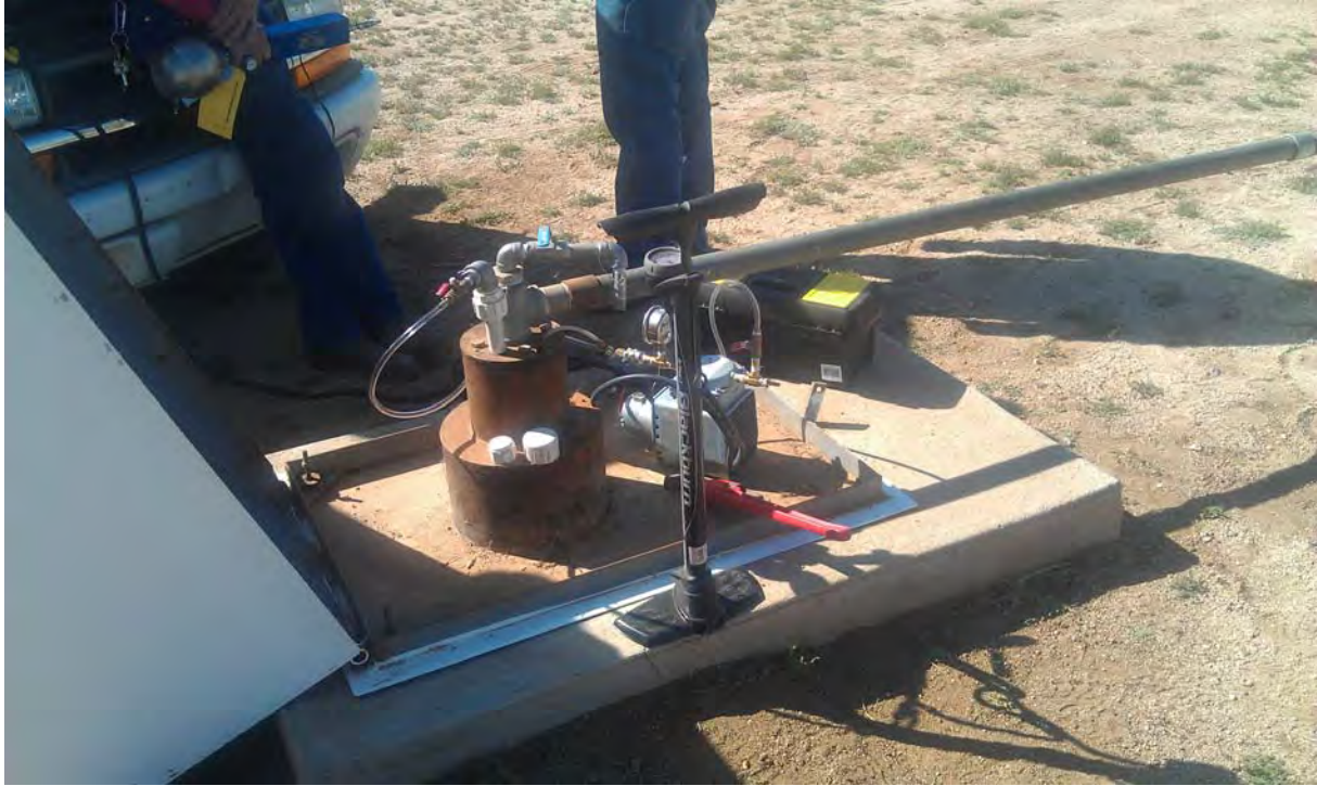
Figure 4. Photograph of retrofitted ground water monitoring well MW-2, while setting it up for soil vapor sampling.
